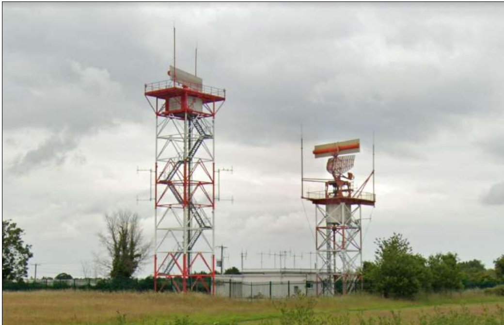
Figure 13. Dublin Airport MSSR Radar Station #2
